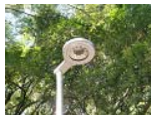
(改修後) LED 99W
